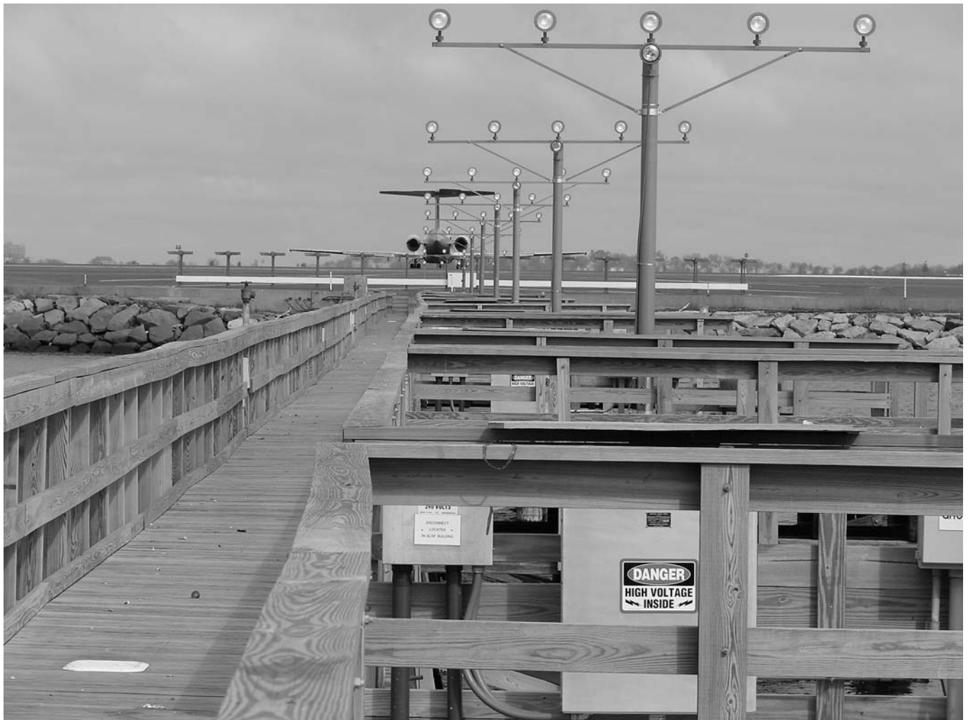
Approach lighting system at Logan International Airport, Boston, MA.
